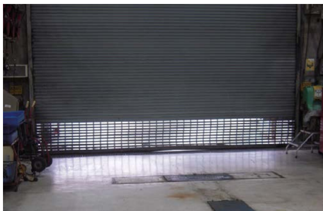
Figure 14. Security mesh in overhead doors. Photo courtesy of Gladstein, Neandross & Associates, NREL 44705
