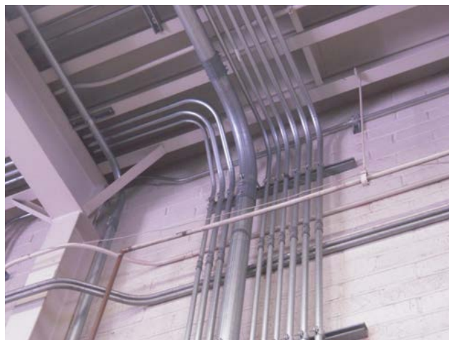
Figure 22. Relocating multiple conduits, such as those shown here, would be costly and complex. Photo from Gladstein, Neandross & Associates, NREL 44676
