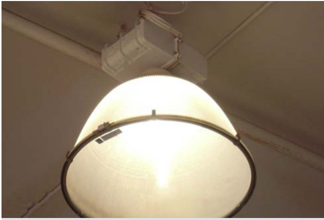
Figure 24. Overhead lighting fixture and ballast that must be relocated. Photo from Gladstein, Neandross & Associates, NREL 44678
