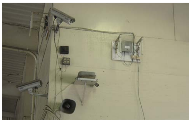
Figure 23. Low-voltage wiring and devices. Photo from Gladstein, Neandross & Associates, NREL 44677
