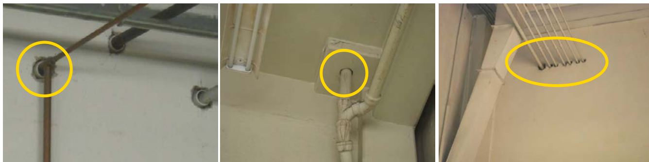
Figure 1. Unsealed conduit or pipes passing through walls or ceilings present a potential path of migration. Photos courtesy of Gladstein, Neandross & Associates, NREL 44893, 44894, and 44895
