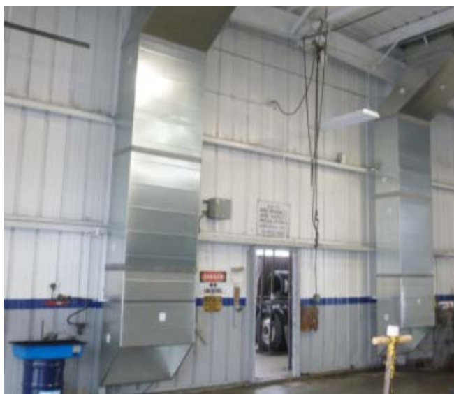
Figure 17. Conventional fuel maintenance facility ventilation pickup points. Photo courtesy of Gladstein, Neandross & Associates, NREL 44699
