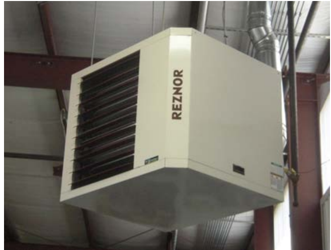
Figure 21. Gas-fired fan heater needs to be replaced or removed. Photo from Gladstein, Neandross & Associates, NREL 44696
