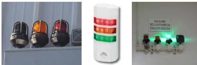
Figure 32. Examples of alarm status lights and horn panels (external and internal). Photo from Gladstein, Neandross & Associates, NREL 44685, 44686, and 44692
